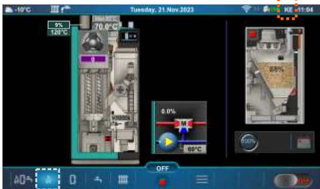
Boiler screen (KE)
