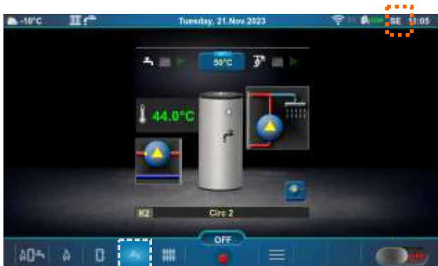
Domestic hot water (DHW) tank screen (SE)
